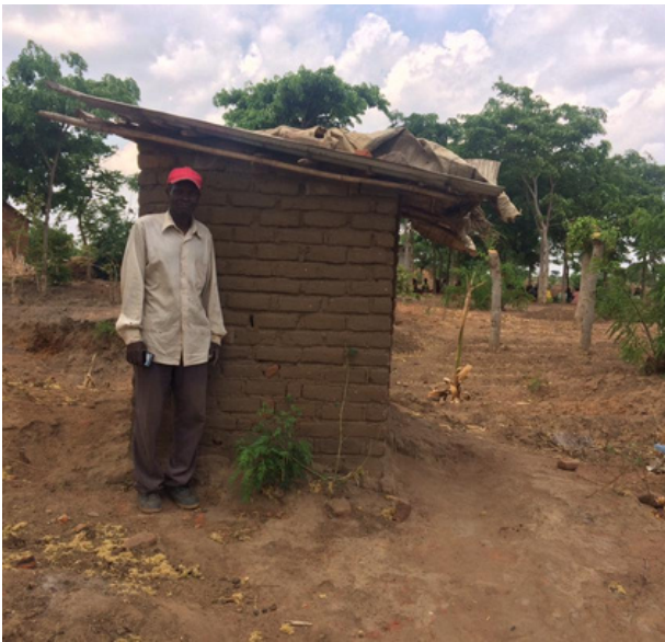
Before | Previous pit latrines
